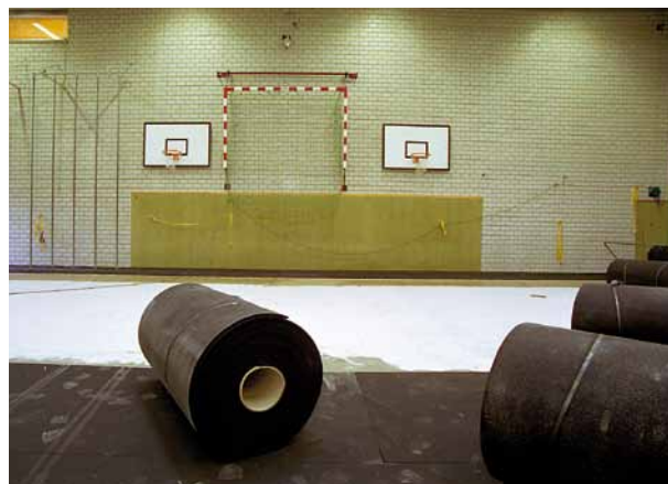
Installing the Regupol® elastic layer. The thickness of the elastic rolls produced by BSW is accurate down to one-tenth of a millimetre.
